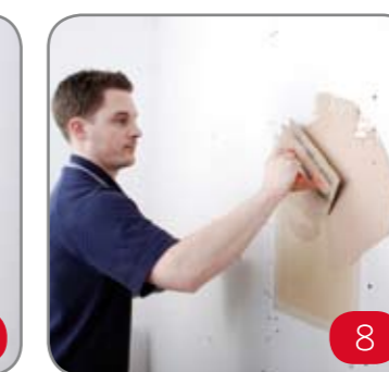
8 Skim with plaster (ordinary multifinish is fine). The best finish is produced when the entire wall is skimmed at the same time.
